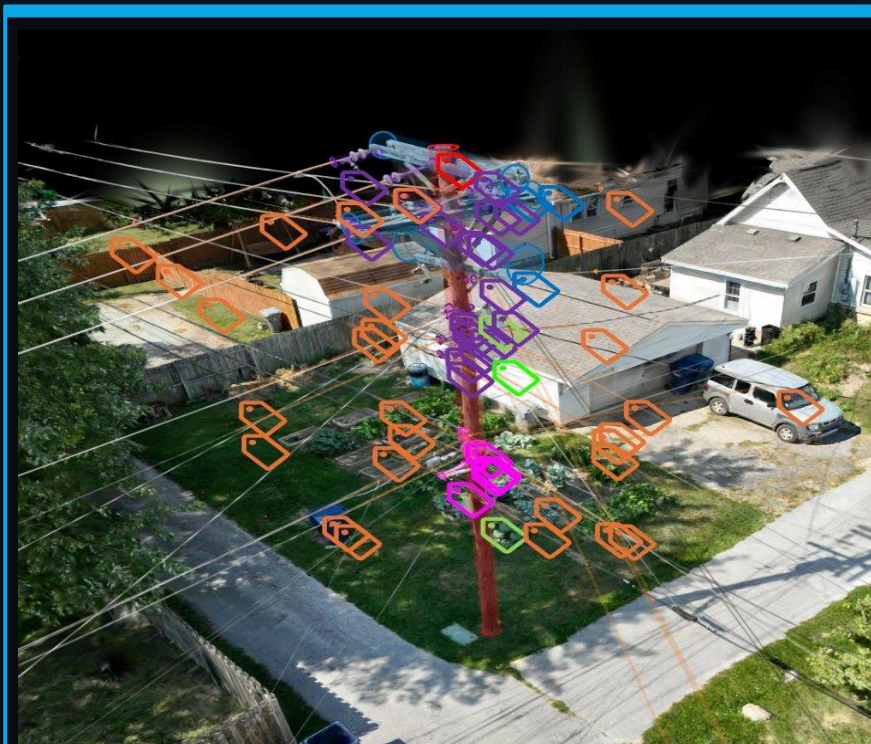
Every component tagged — cross arms, insulators, wires, hardware
